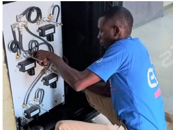
An ETS telecommunications officer fixes critical equipment in the Security Operations Centre (SOC) in Damaturu.
