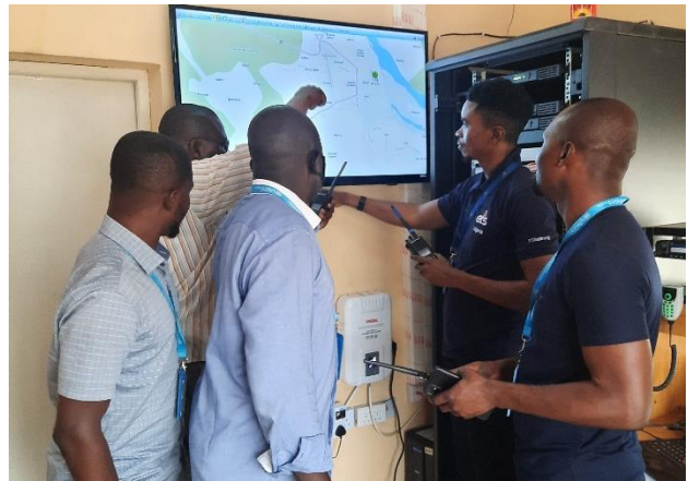
ETS telecommunications staff train UNDSS Security Operations Centre (SOC) operators in Yola.
