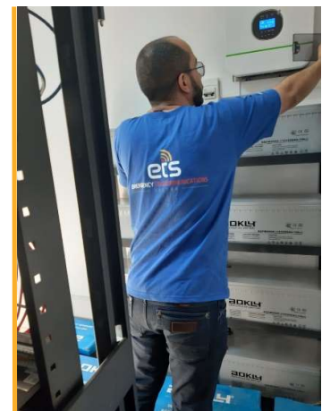
ETS upgrades equipment in the Security Operations Centre (SOC) in Benghazi. Photo: WFP/ETS
