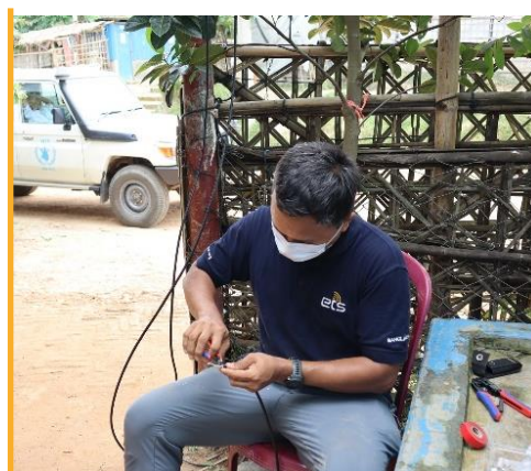
The ETS connecting the IOM Liquefied Petroleum Gas (LPG) in Camp 20 extension to the ETS network. Photo: WFP/ETS
