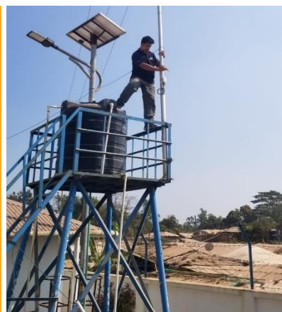
The ETS realigning the radio link mast for improved signal strength in Leda. Photo: WFP/ETS
