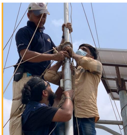
ETS installs new equipment in Teknaf to upgrade the network in surrounding sites. Photo: WFP/ETS
