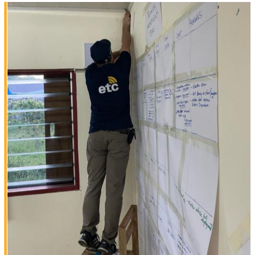
The ETC installing data connectivity at Tafea PEOC in Tanna. Photo: WFP/ETC
