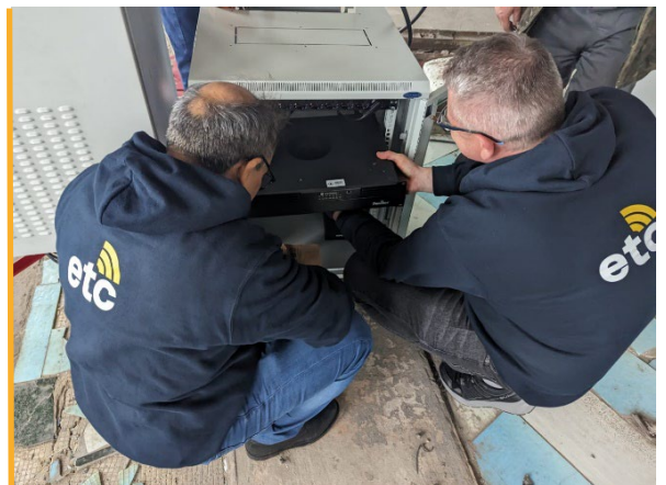
The ETC specialists install VHF radio repeater in Kyiv on 25 October to expand radio coverage in the city. Photo: WFP/ETC
