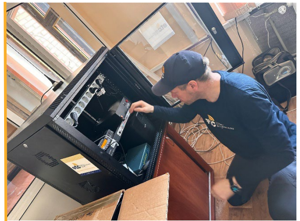
The ETC on mission in Kramatorsk on 19 September to debug the faulty VHF radio equipment. Photo: WFP/ETC
