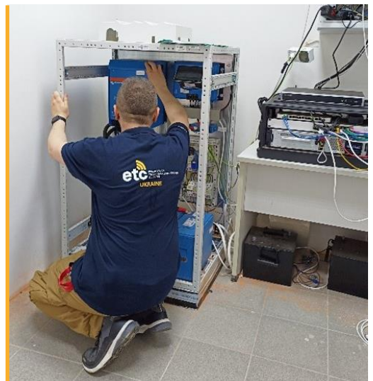
ETC visits UNDSS to support the Security Information Operation Centre (SIOC) and check power supply equipment. Photo: WFP/ETC
