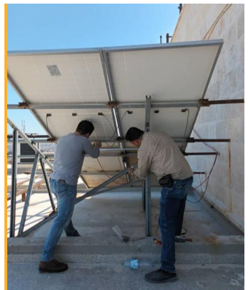
The ETC resolved solar power issues at the UN hub in Aleppo in April. Photo: WFP/ETC
