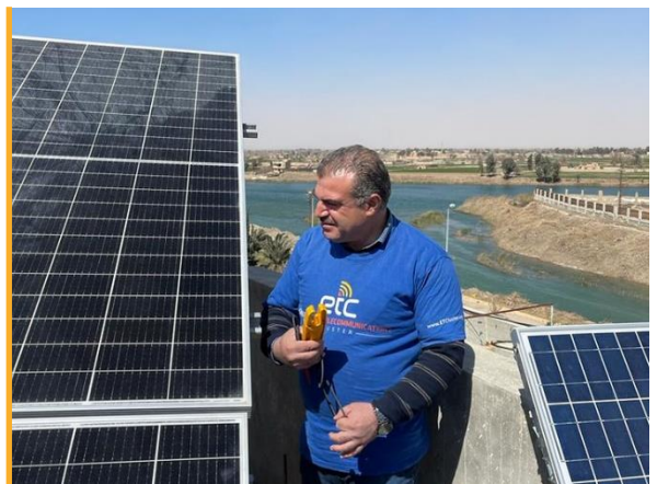
The ETC is carrying out maintenance and improvement activities across five UN hubs in Syria. Photo: WFP/ETC
