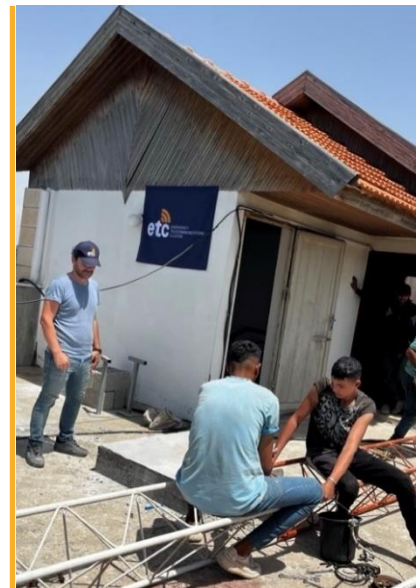
The ETC installs a VHF radio repeater mast in Deir Al Balah, Gaza. Photo: WFP/ETC
