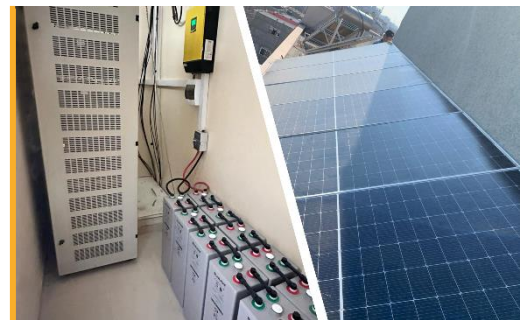
The ETC supported solar power solution installation at the VHF radio repeater site in Rafah, Gaza. Photo WFP/ETC
