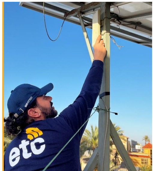
The ETC tests the VHF radio repeater at Al Shaboura Clinic in Rafah, Gaza. Photo: WFP/ETC
