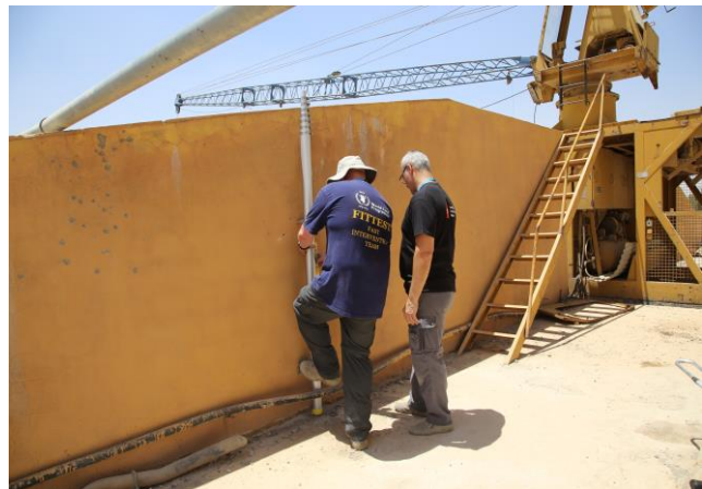
The ETC team is setting up security telecommunications services and Internet connectivity in Adha IHP camp. Photo: WFP/ ETC Iraq
