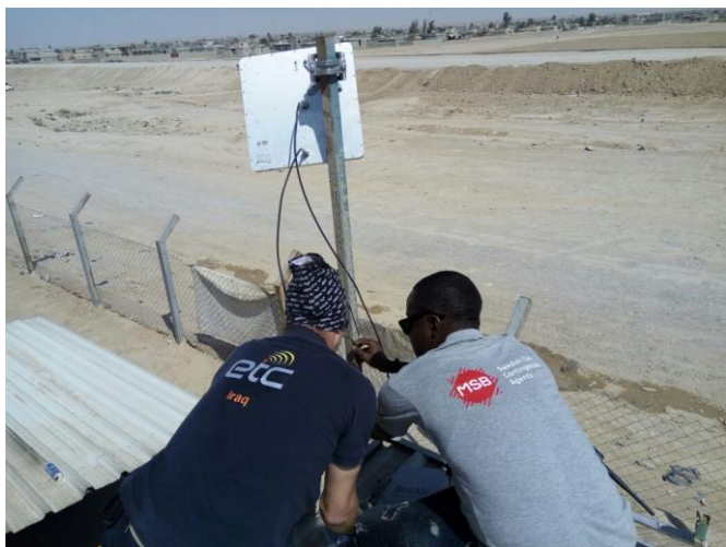
The ETC team setting up equipment from the ETC member Ericsson Response in Jeddah camp 1. Photo: WFP/ ETC Iraq
