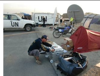
Installation of the mesh network delivering voice and data services at the UN compound in Port Au Prince
