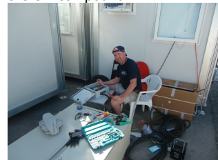
John Jeffries, Irish Aid, building the electrical network in the Port Au Prince camp.
