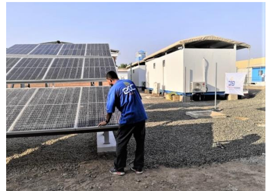
A member of the ETC team checks a solar panel installed at the UN hub in Al Mokha. Photo: WFP/ETC
