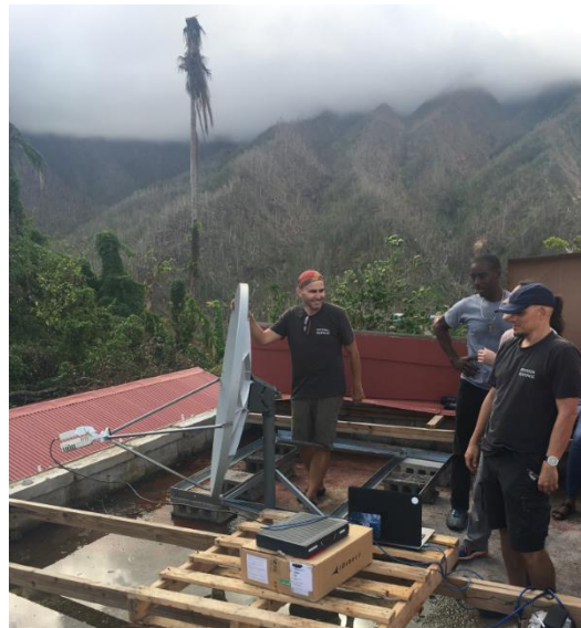
The ETC is supporting the government with the installation of a new satellite terminal in Delices, Dominica. Photo: Débora Natareno/WFP
