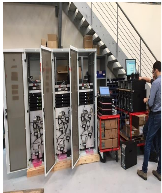
Configuration and testing of Digital Mobile Radio network infrastructure in Denmark.
