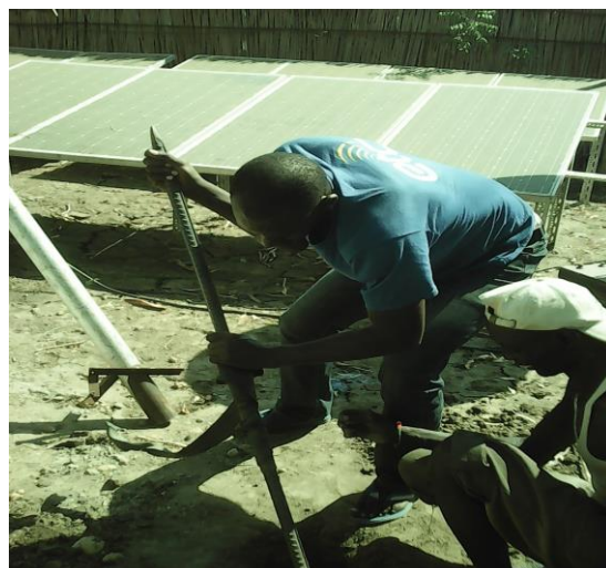
Repeater for the security telecommunications supported by renewable energy solution installed. Ganyiel, South Sudan
