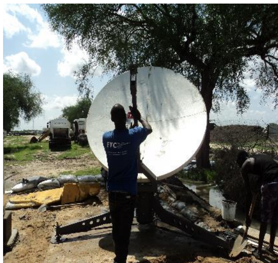
Ku-band Communication Satellite Antenna installed in Pibor, South Sudan
