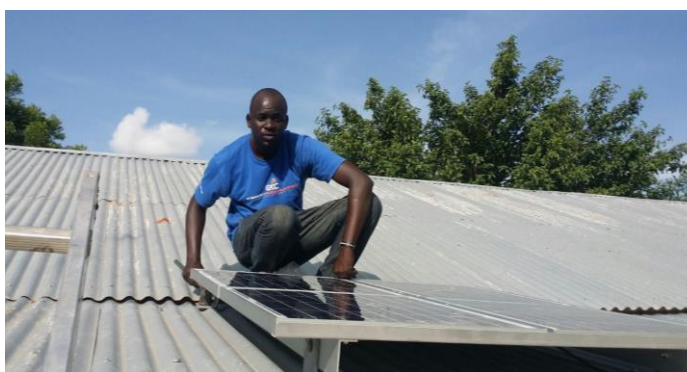
ETC technician, Loro Wani, installing solar panels to power the Internet service for humanitarian in Akobo (Jonglei state) Photo: ETC
