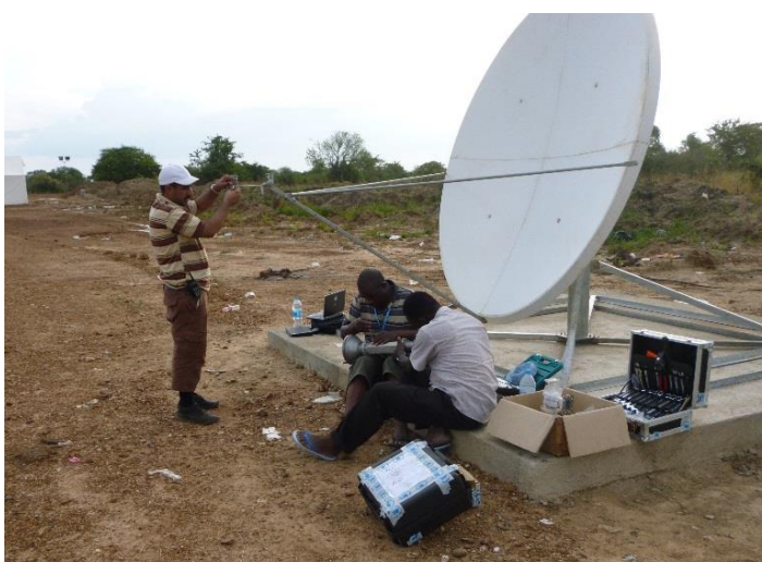
ETC and WFP Technicians Tenson Majaraunga, Khalid AlZaba and Martin Hakim performing VSAT installations in Mingkaman (Lakes State), Photo: WFP/ Zacharia Yasir
