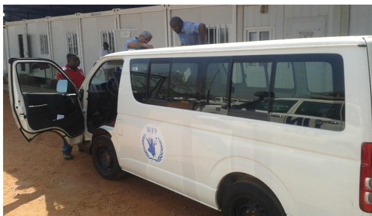
Installing a VHF radio transmitter on a WFP van (Juba). Photo: WFP/Simone Alzari
