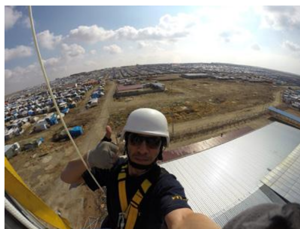
An ETC telecommunications specialist installing a radio antenna on top of the mast at Domiz camp. Photo: WFP/Fabrice Bouguerra
