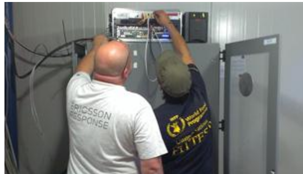
FITTEST and Ericsson Response staff installing WIDER equipment at Domiz camp to extend ETC wireless connectivity.
