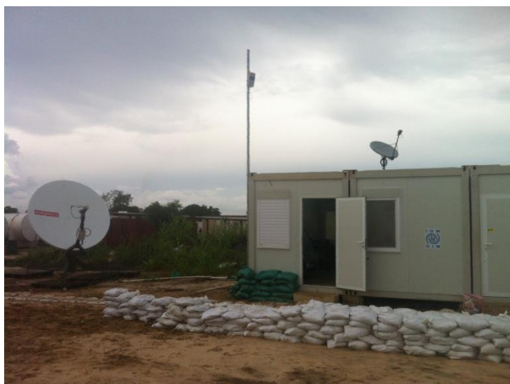
The ETC Response Solution installed in Bentiu (Rubkona). Photo: WFP/John Mawa
