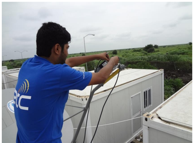
Installing the k-band VSAT in the new humanitarian hub in Malakal, Upper Nile state. Photo: DishNet/ Hardik Rajesh Kumar
