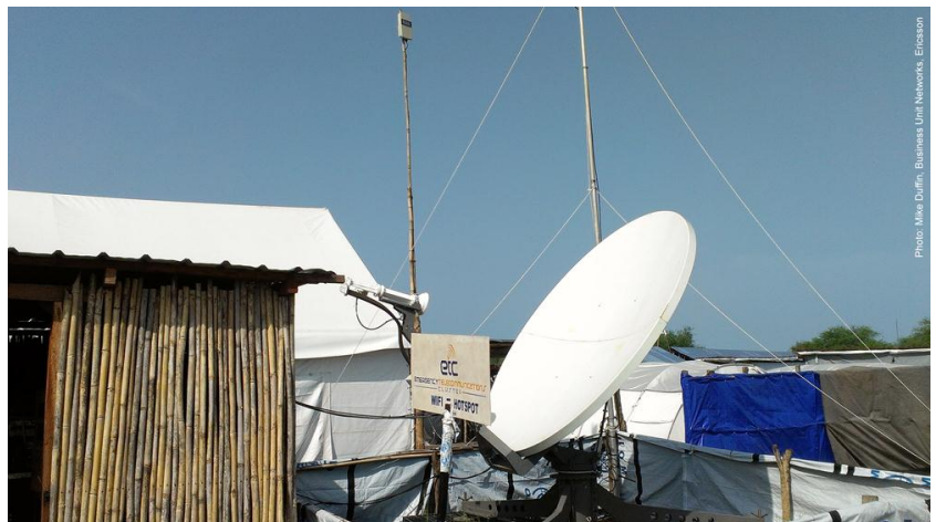
ETC Voice and Data solution, with equipment from emergency.lu and Ericsson Response, in Mingkaman, Lakes State.
