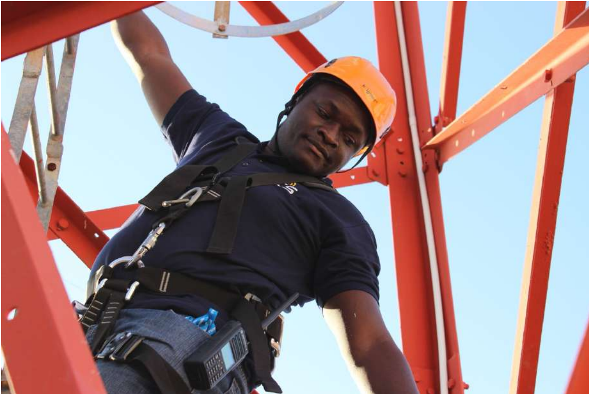
Photo Credit: Emergency Telecommunications Cluster
